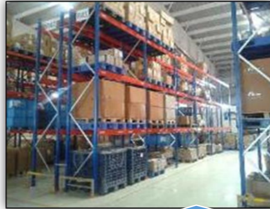
High Bay Racks in Central WH -Construction & Space Savings by 2x
